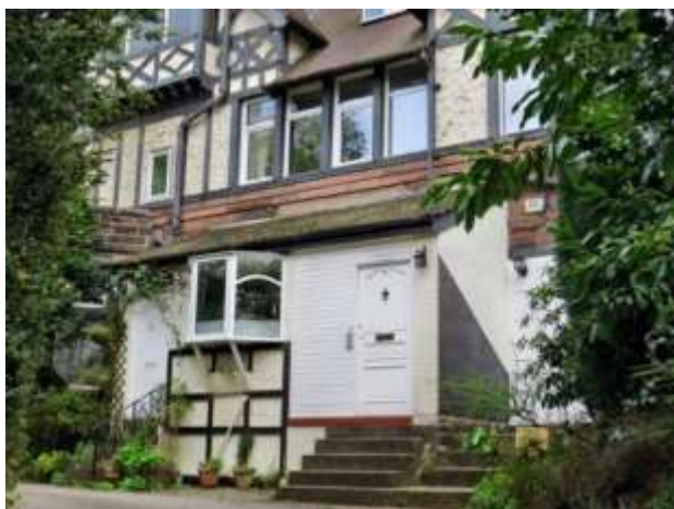
Flat conversions on Stamford Road, where the creation of multiple entrances has not been sympathetically designed to suit the character of the building
